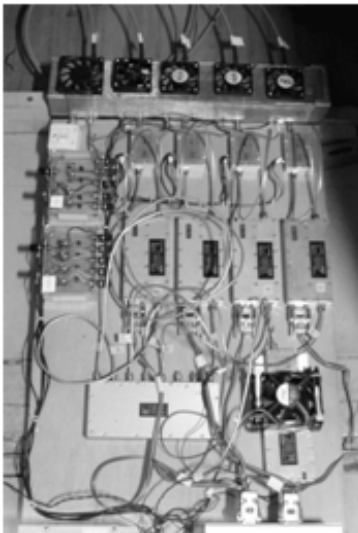
Fig. 3. The picture of the antenna array system.
